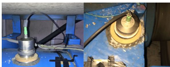
Fig. 2. Accelerometers for LSS (left) & HSS (right)
